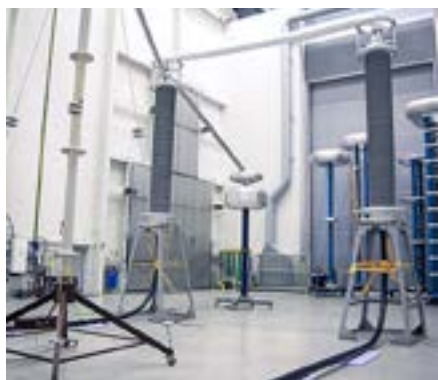
Several test halls for testing at different voltage levels.
